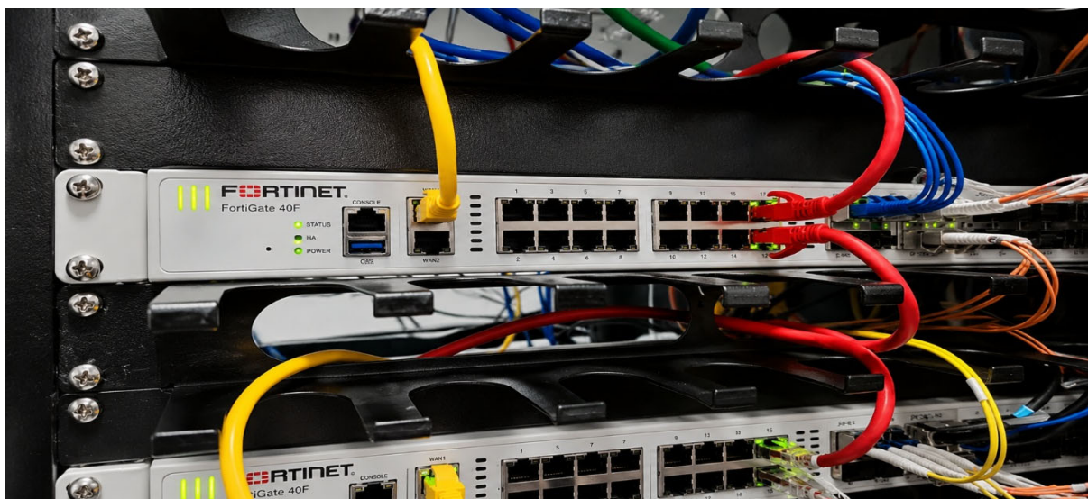
Figura 10 - Firewall Fortinet – Fortigate 400F.
